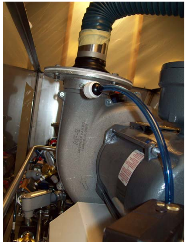
Air/Particulate Sample near exhaust using ESA Filter Cartridge.
